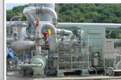
Fuel Gas Compressor
